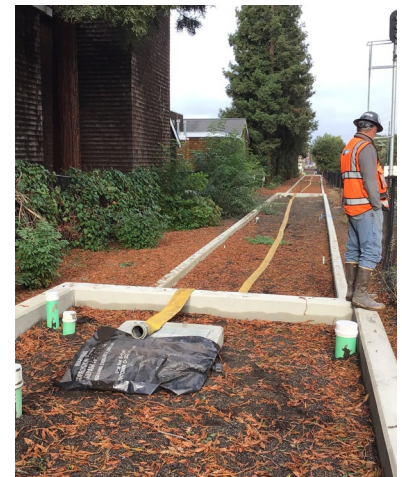
Bioretention Area Drainage
